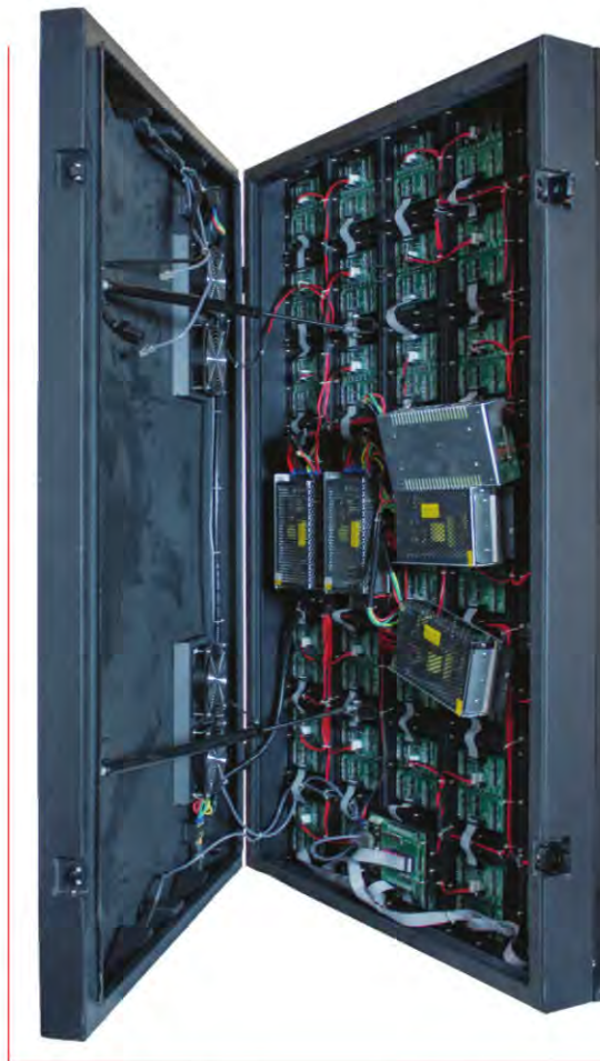
Many cabinet-style LED signs feature only one transformer, long, exposed cables and blowing fans, all of which reduce energy efficiency.
